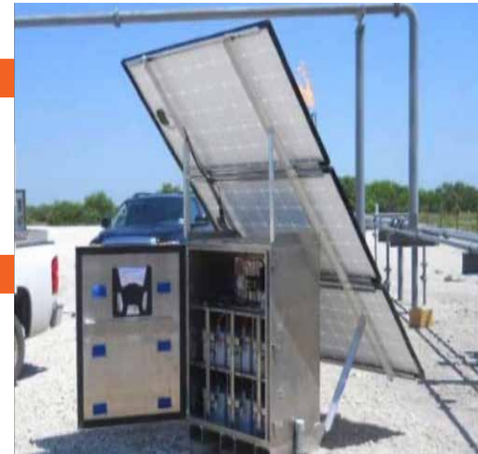
SunSavers in remote powering system by Deka Solar and Ameresco, Eagle Ford Shale site in Texas
