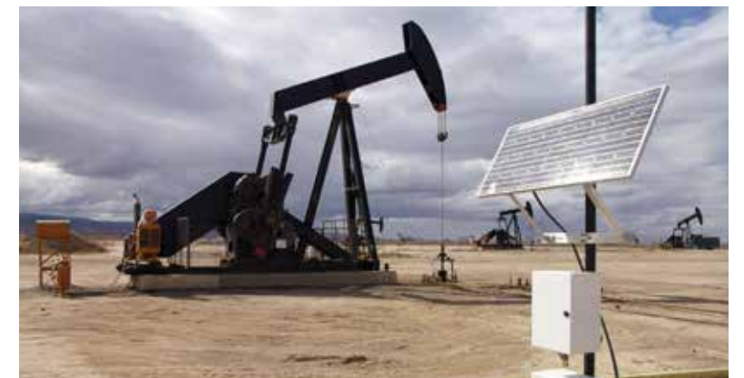
Remote oilfield solar installation with the Morningstar SunKeeper on-board. Courtesy SunWize
