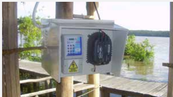
SureSine inverter being used in a tropical marina dock-side power application
